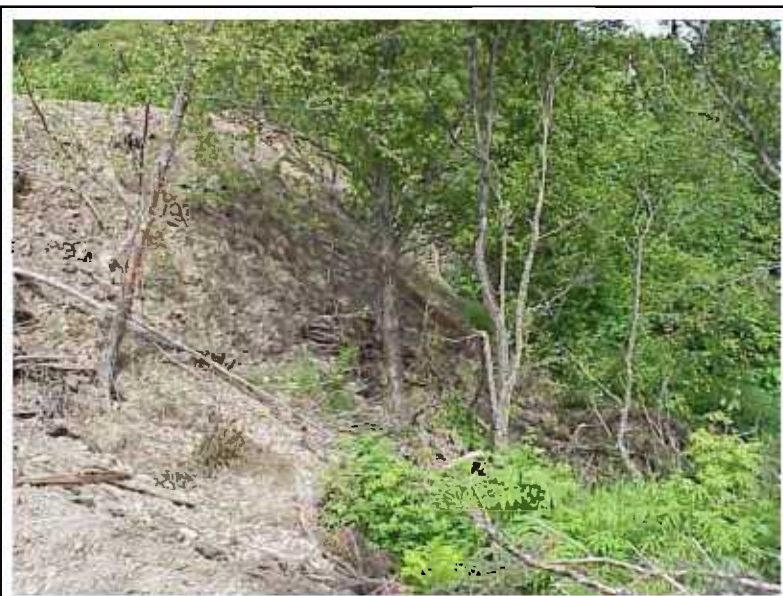
Fill Eroding Over Side of Parking Lot at Hornaday Park
