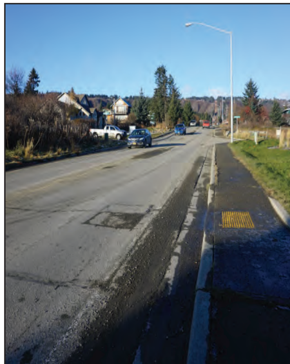
Photo showing the beginning of soft spots mid-way down Heath Street.
