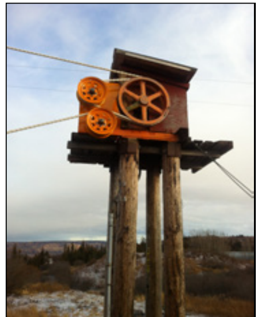
Ohlson Moutain Rope Tow's top station, which supports the engine, bullwheel and weight of the rope in motion, is in need of foundation repair.
