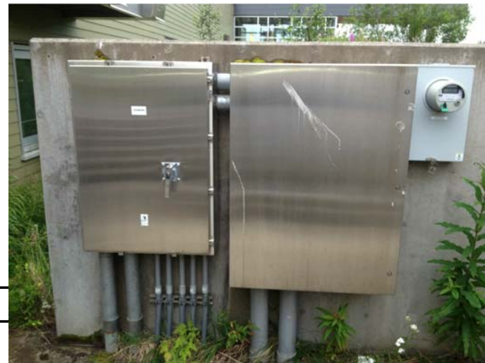
EXISTING ELECTRICAL PANELS
