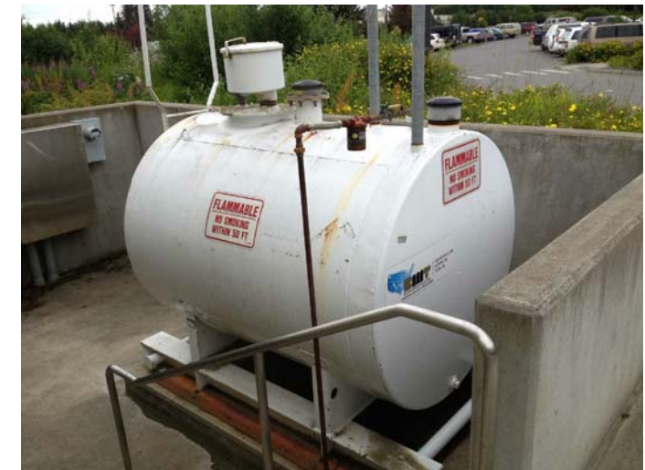
EXISTING FUEL TANK AND FUEL LINE
