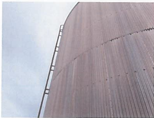
Side View Tank
