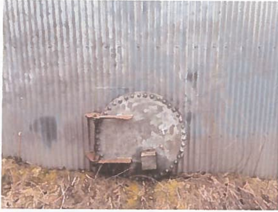
Tank Access Hatch
