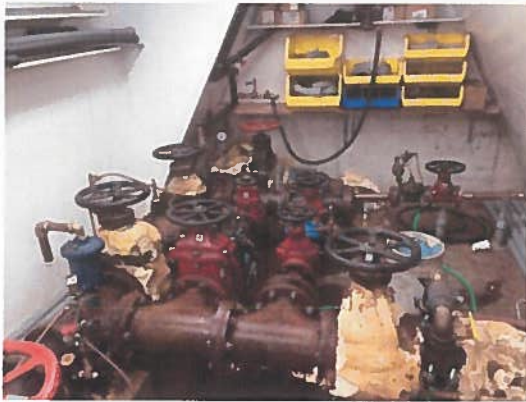
Valves in Mechanical Building
