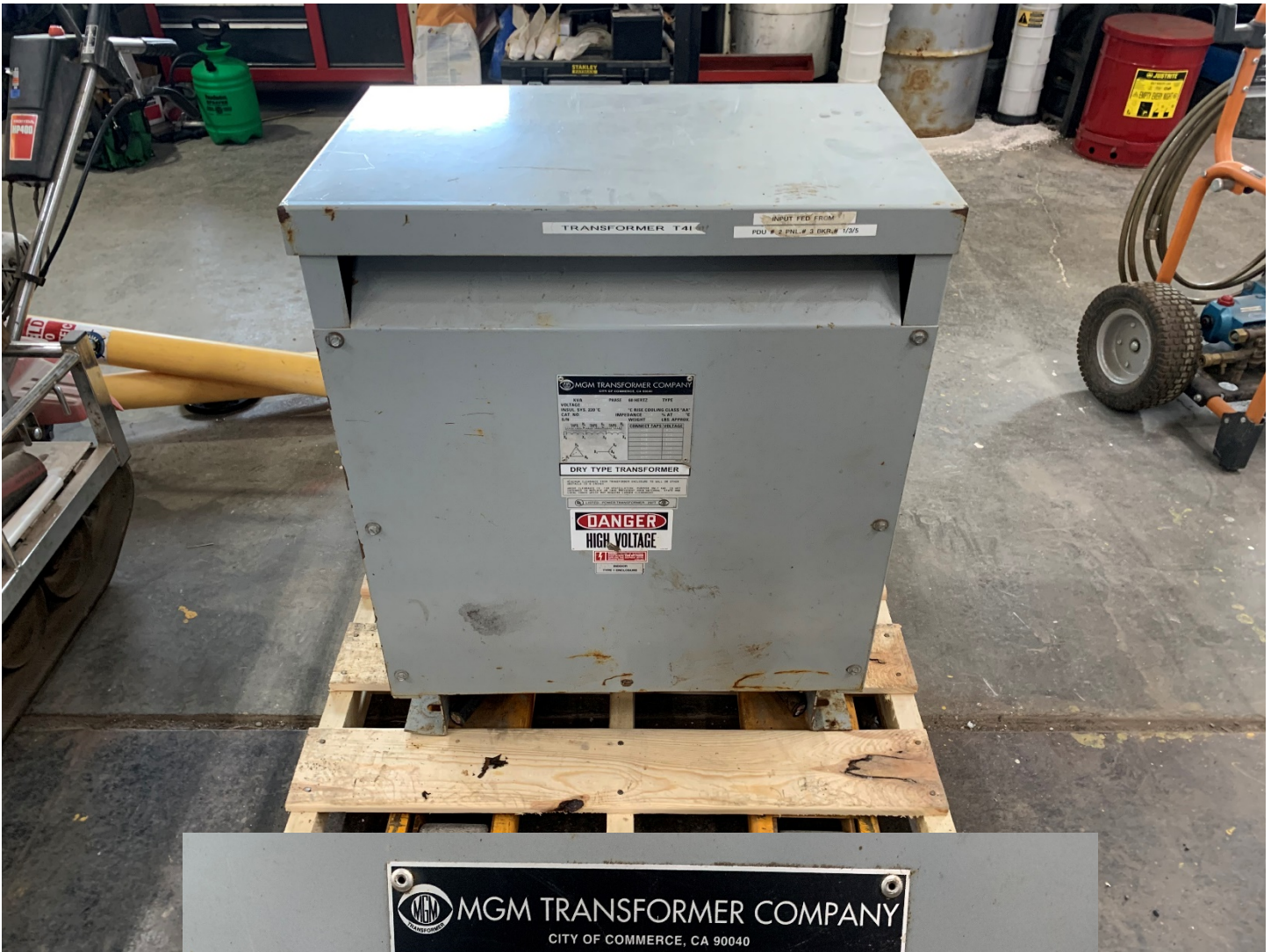
Item #3 Isolation Transformer, MGM Transformer Company, Cat#AD370-E039
