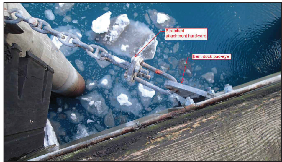
2 TYPICAL ATTACHMENT HARDWARE DAMAGE
