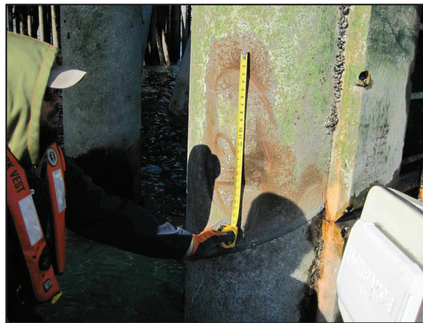
4 SOUTH SLEEVE DAMAGE TO FENDER 15
