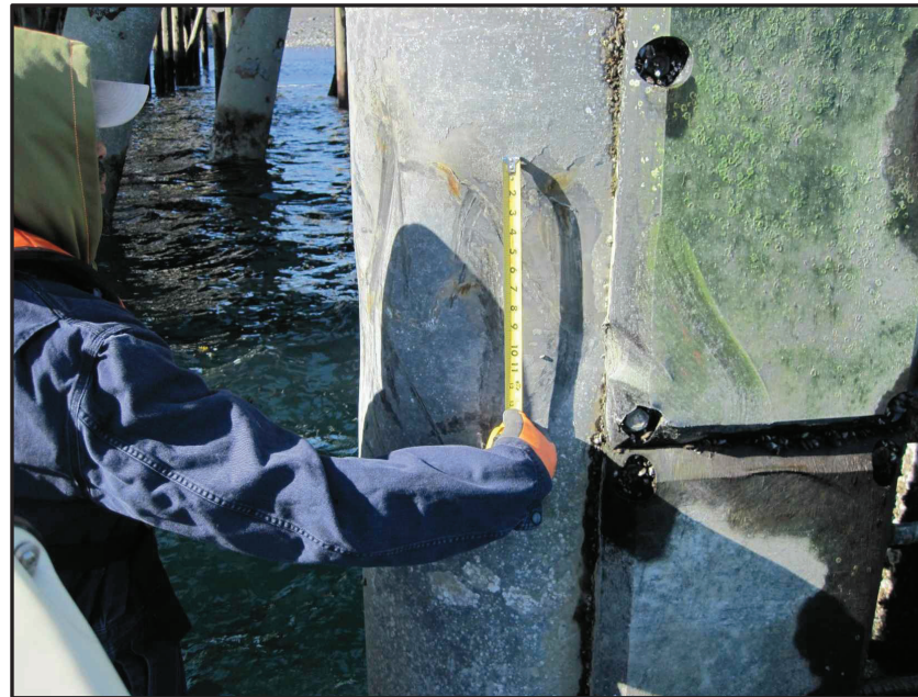
3 SOUTH SLEEVE DAMAGE TO FENDER 14
