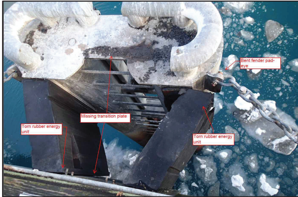
1 TYPICAL FENDER DAMAGE
