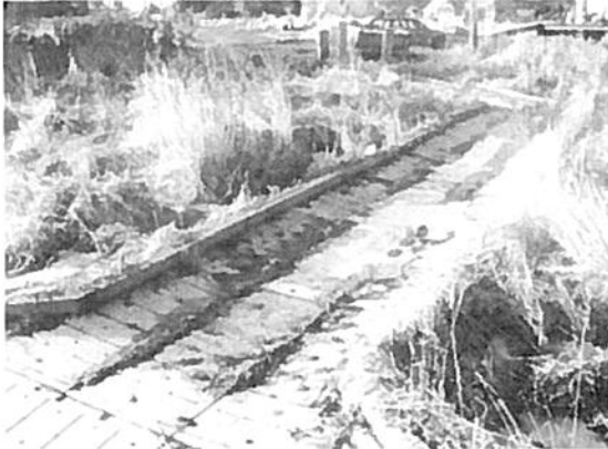
Figure 1 -- Deteriorated Trail Damaging Wetlands
