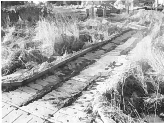
Figure 1 -- Deteriorated Trail Damaging Wetlands
