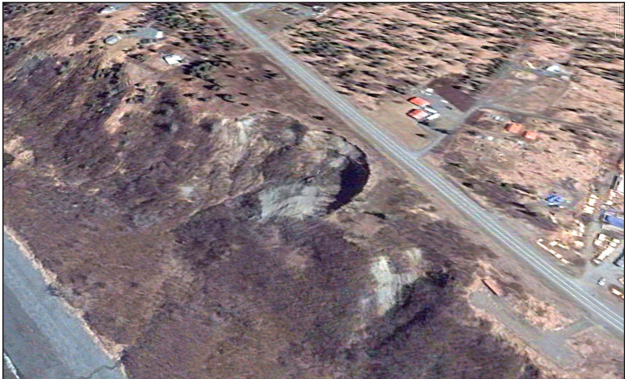
As seen in this aerial image, the eroding edge of the bluff is only 30 feet away from the Sterling Highway at a section just north of Anchor Point.
