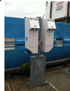
New Electrical Pedestal
