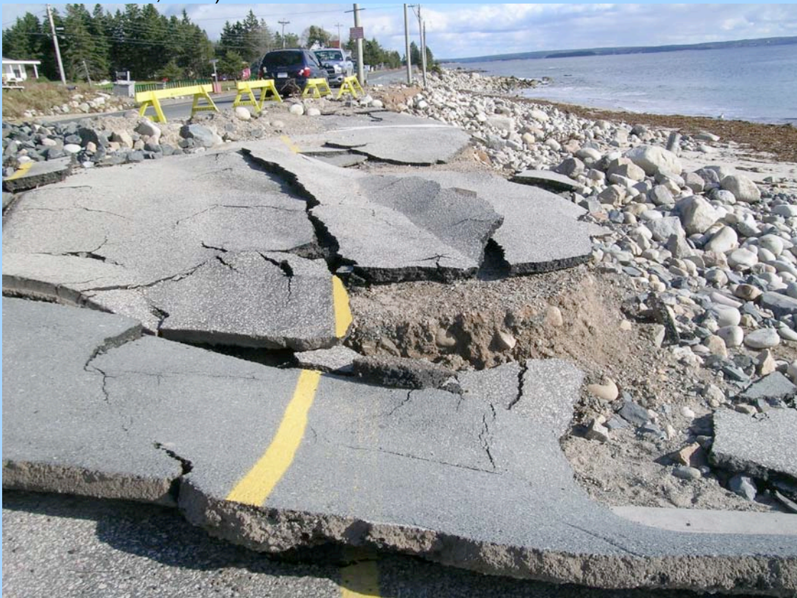
Figure 4.12. Road damage adjacent to Queensland Beach after a 2007 storm. Photo courtesy of A. Baccardax.
