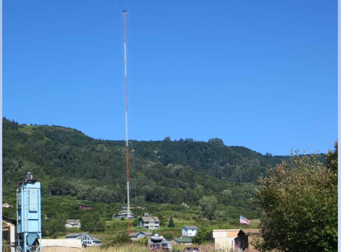
275 ft. “guyed” tower Kachemak City
