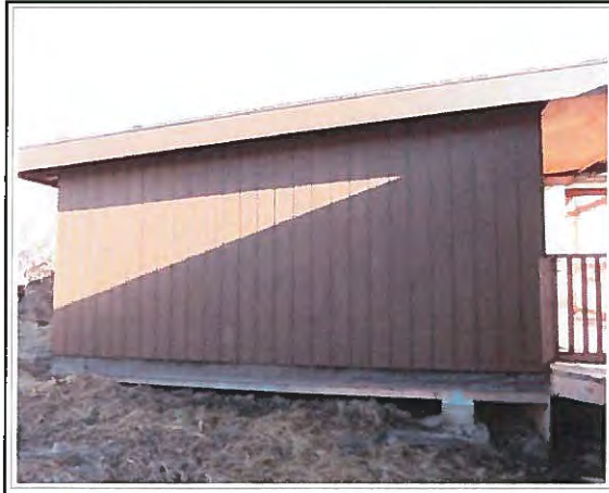
The 12' x 18' storage shed between Cabins 4 and 5. This was added since March, 2013.
