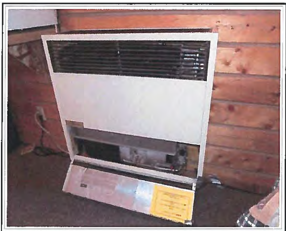
Cabin 1 LP-gas unit heater
