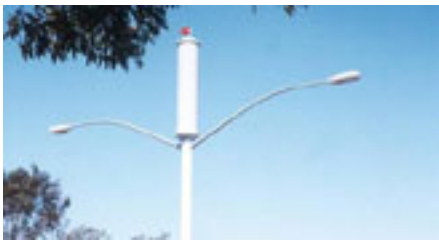
✚ Figure 7 Antennae on Parking Light Stand
