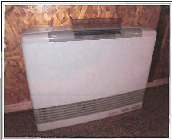
Cabin 4 LP-gas unit heater
