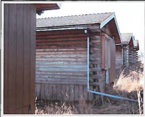
Looking south at the rear of the west cabins. The rear and sides of the cabins could use surface preparation and new oil or stain.
