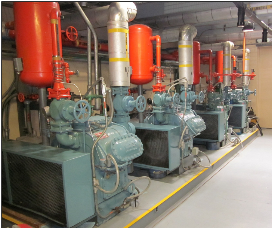
Four of the Ice Plant's aging compressors are shown here.
