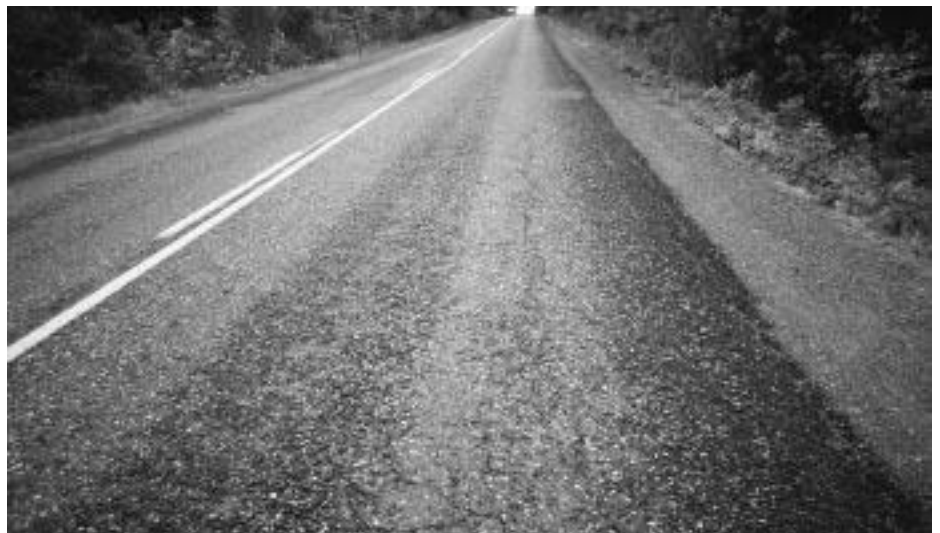
► Moderate to severe raveling in wheel paths.
