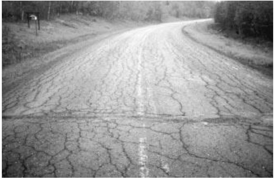
▶ Extensive alligator cracking. Pulverize and rebuild.
