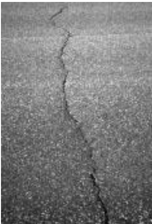
▲ Tight cracks less than 1/4" in width.
