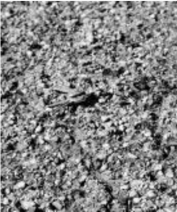
Severe raveling with ▼ extreme loss of aggregate.
