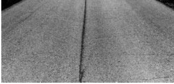
Edge cracking from weakened subbase and traffic loads. ▼
