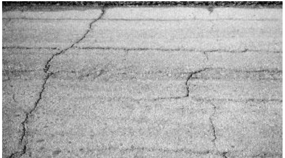
▼ Block cracking with open cracks.
