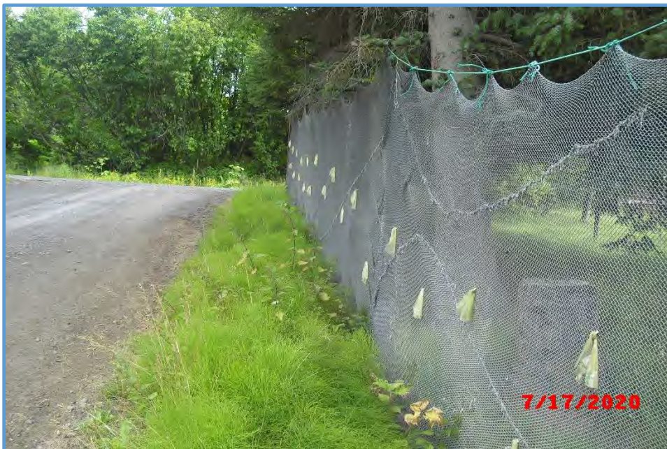
Figure 10: Spruce trees in corridor preventing proper ditch establishment
