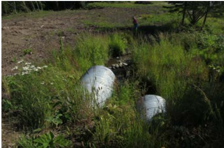
Pioneer Avenue culvert outlet. Source: Lisa Holzapfel.
