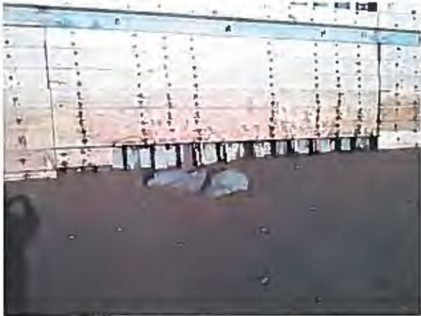
Typical maintenance issue - erosion at toe of wall
