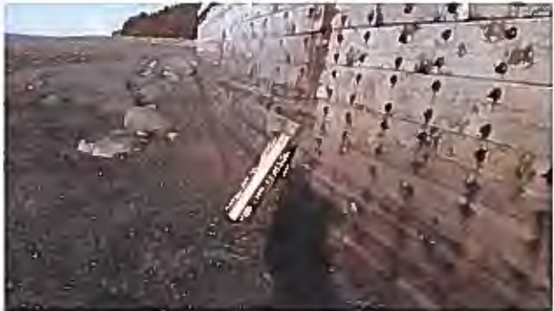
Timber face damage - repaired in 2016
