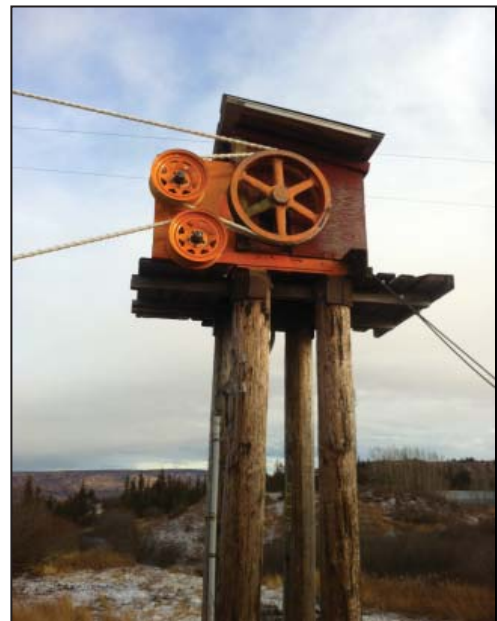
Ohlson Mountain Rope Tow's top station, which supports the engine, bullwheel and weight of the rope in motion, is in need of foundation repair.
