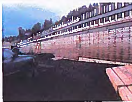
Typical maintenance issue - erosion at toe of wall - extended wood face lower
