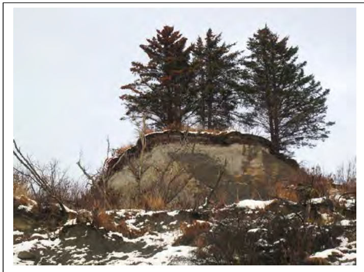
Looking up from the beach, chunks of land slough downward toward the shoreline.
