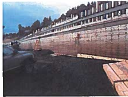
Typical maintenance issue - erosion at toe of wall - extended wood face lower
