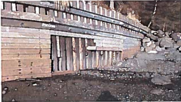
Unusual - but lost almost two entire panels in February
