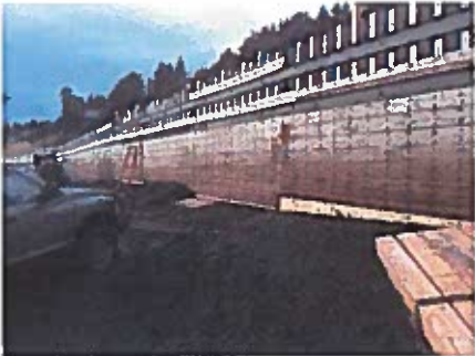
Typical maintenance issue - erosion at toe of wall - extended wood face lower
