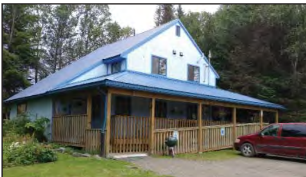
Annual maintenance to the Annex, an older, former residential building that houses several SPBHS programs, often exceeds SPBHS' entire agency maintenance budget.
