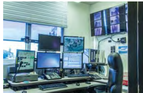
City-wide radio system upgrades are needed to maintain full communication operability.
