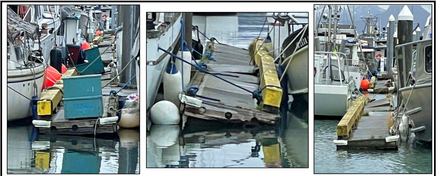
Figure 2.29: Tee floats, located along the harbor channel, are broken and severely listing.
