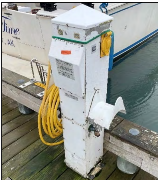
Figure 2.18: Power/water pedestal coating damage
