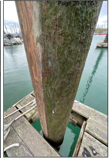
Figure 2.46: Moderate wear on timber piles.
