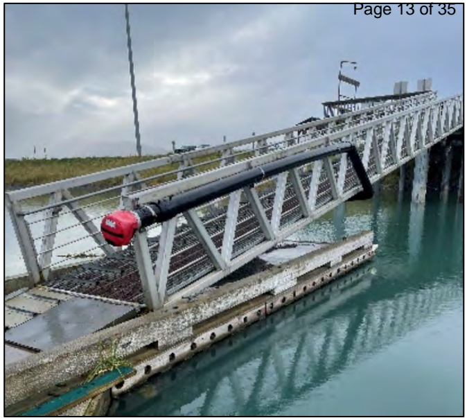
Figure 2.13: Fire system HDPE piping on Ramp 4.
