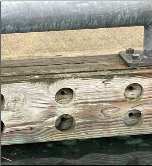
Figure 2.22: Missing through rods.
