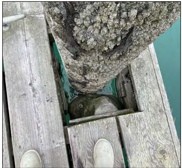
Figure 2.47: View under deck at a pile location. The odd shaped grey item floating between the pile and persons foot is very deteriorated flotation foam that is loose.
