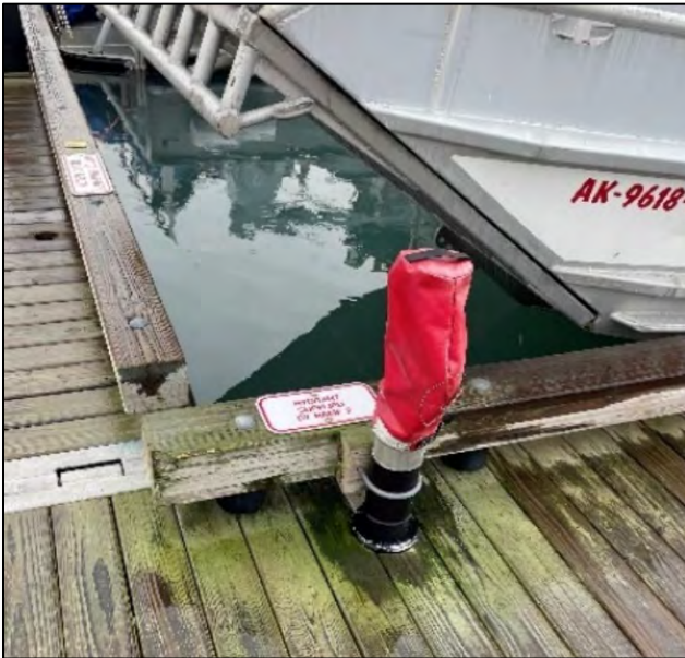
Figure 2.12: Fire suppression system standpipe/hydrant near J Float
