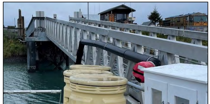
Figure 2.17: HDPE fire suppression piping at Ramp 2
