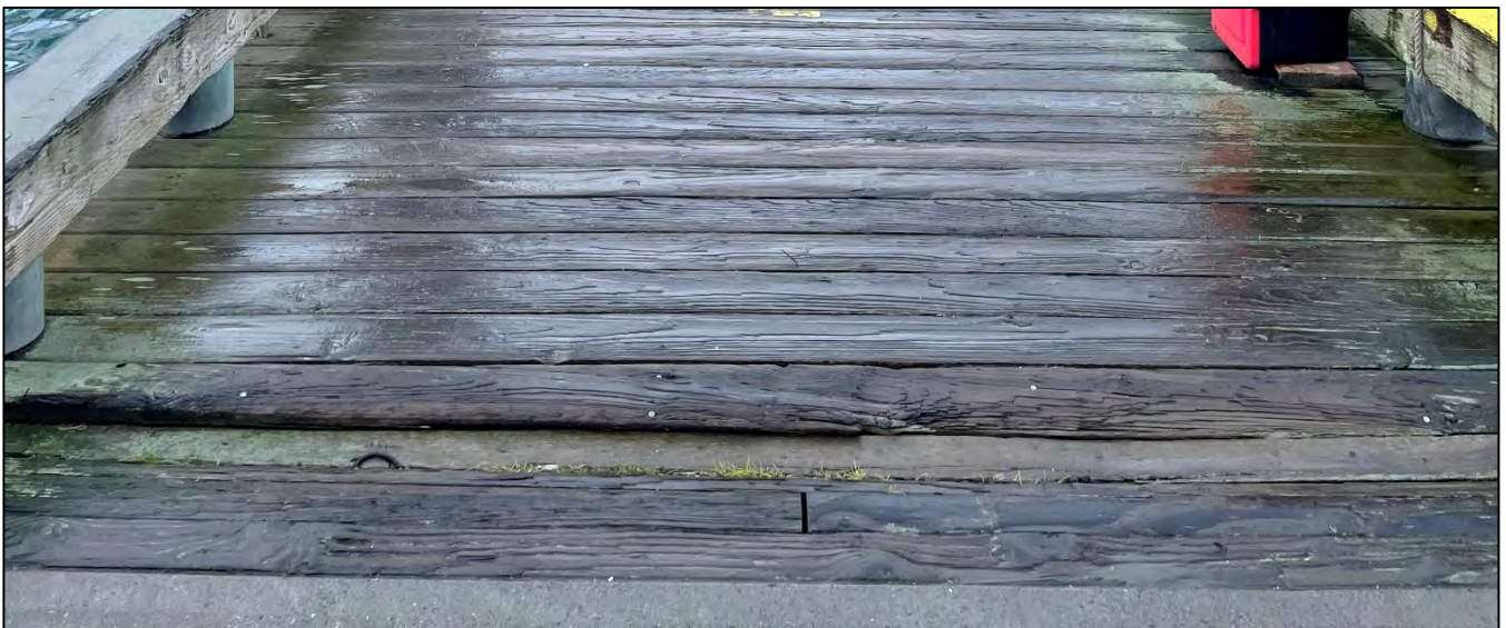
Figure 2.14: Typical decking wear at high traffic areas (float intersections)
