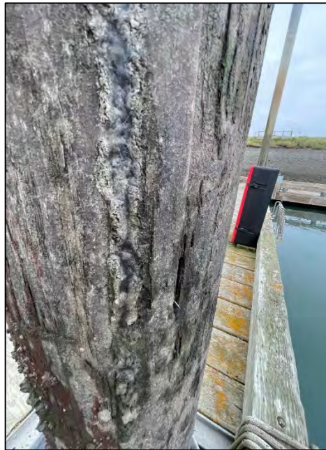
Figure 2.45: Timber pile with advanced deterioration/rot
