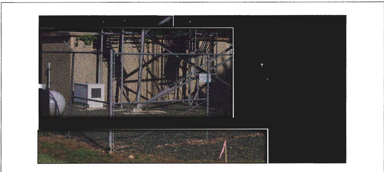
Figure 2: Example of 800 MHz Base Station
