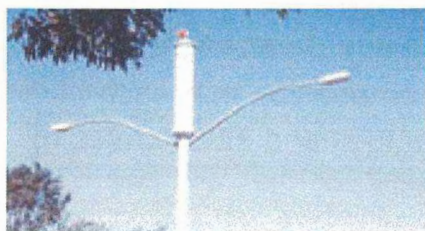
▣ Figure 7 Antennae on Parking Light Stand
