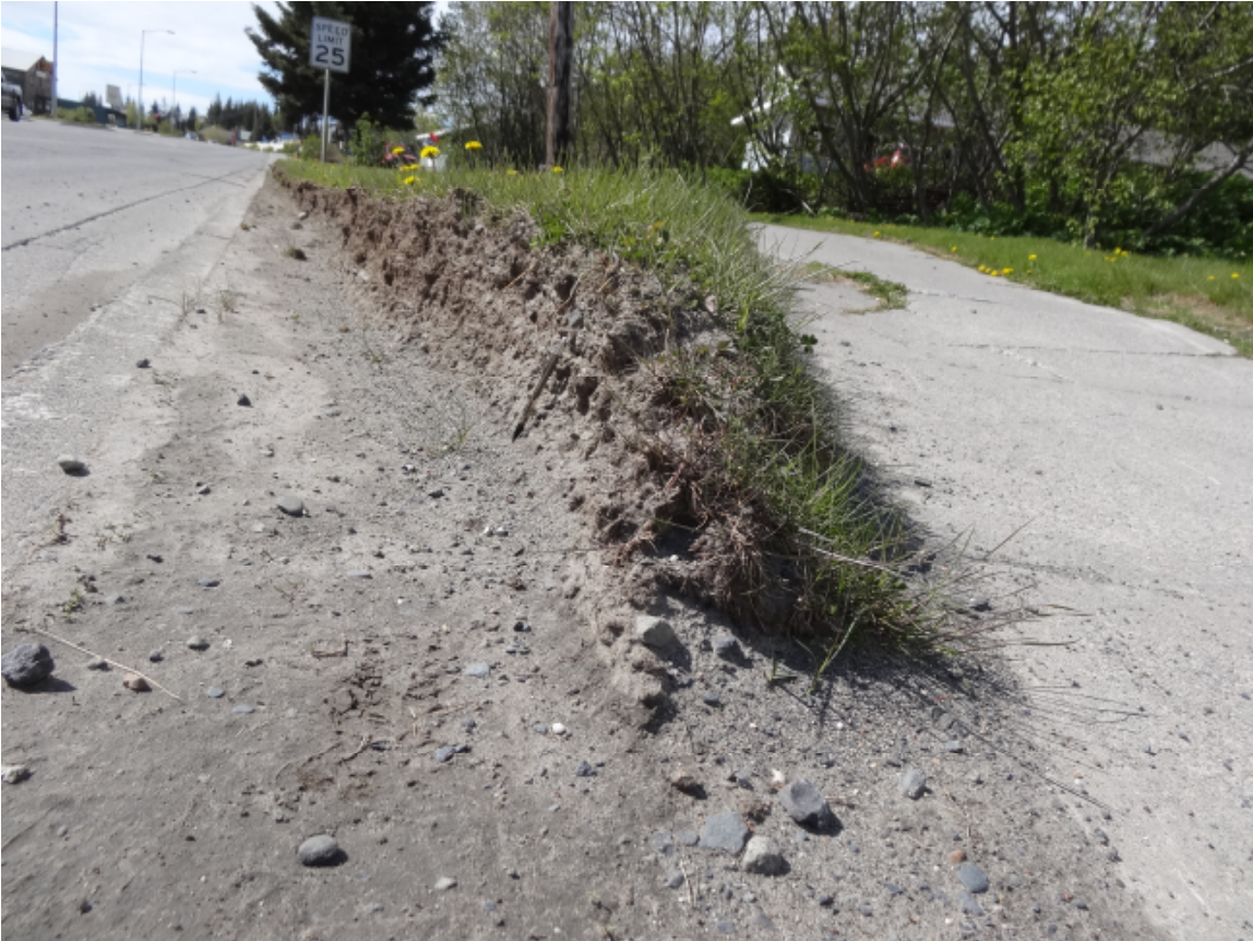
Pics of raised sod between curb and sidewalk on north side of Pioneer in front of Borough office (206 E. Pioneer)
