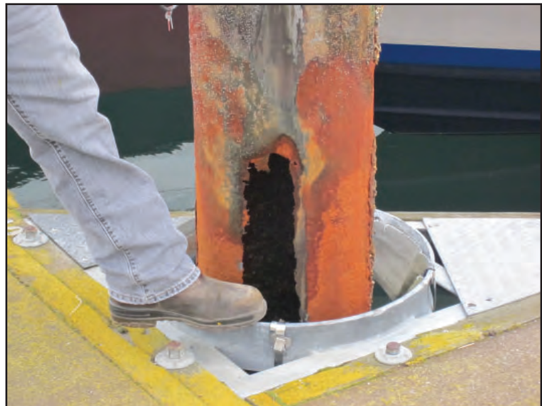
Example of the damage electrolysis causes to harbor pilings. This broken piling in 2012 caused the R & S floats in the harbor to be condemned until it could be repaired.
