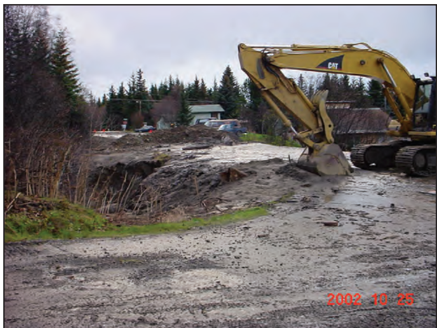
A master plan is needed to address storm water management issues.
