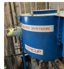
Teacup: grit-removal filtration system.
