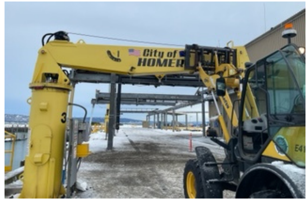
Forklift getting in place to support the crane boom for the repair.
