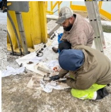
Jedidia Gautier, (yellow pants) and James Young in ball cap making repairs.
