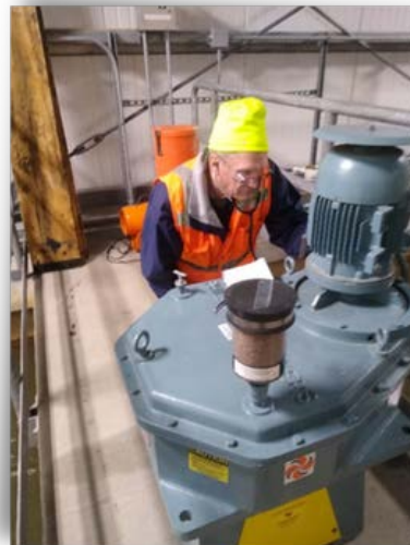
John Koch listens to a mixer in the water treatment plant with a stethoscope. This was done for every machine with a motor.
