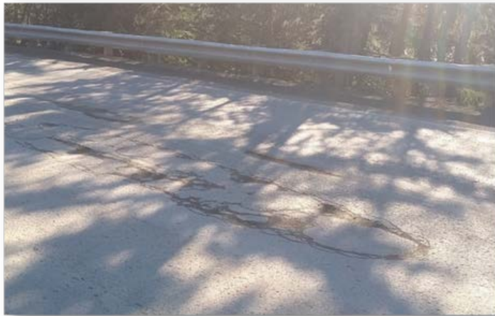
Pothole damage on East Hill Road
