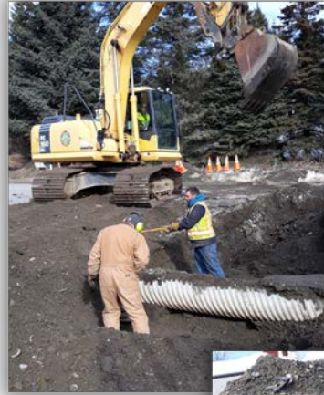
Left: Crew backfilling trench after repairing the sewer service line on Kachemak Way.
