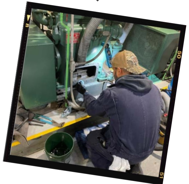
James Young services a compressor.
