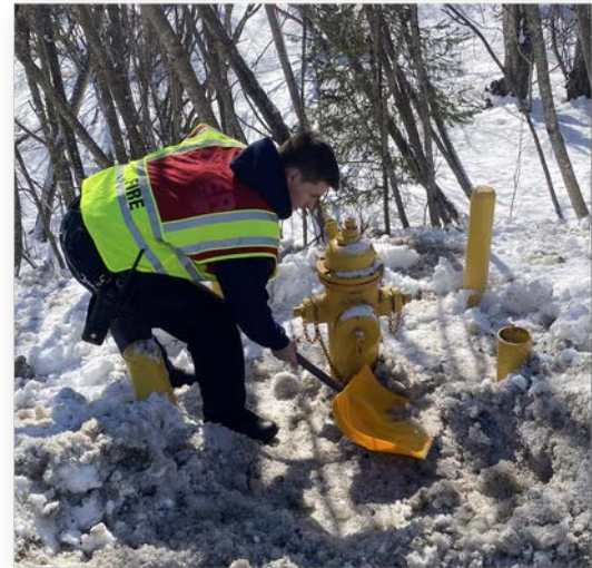
HVFD friendly reminder to help clear the snow away from your hydrants. Pictured above: Firefighter/EMT Lowe hard at work
