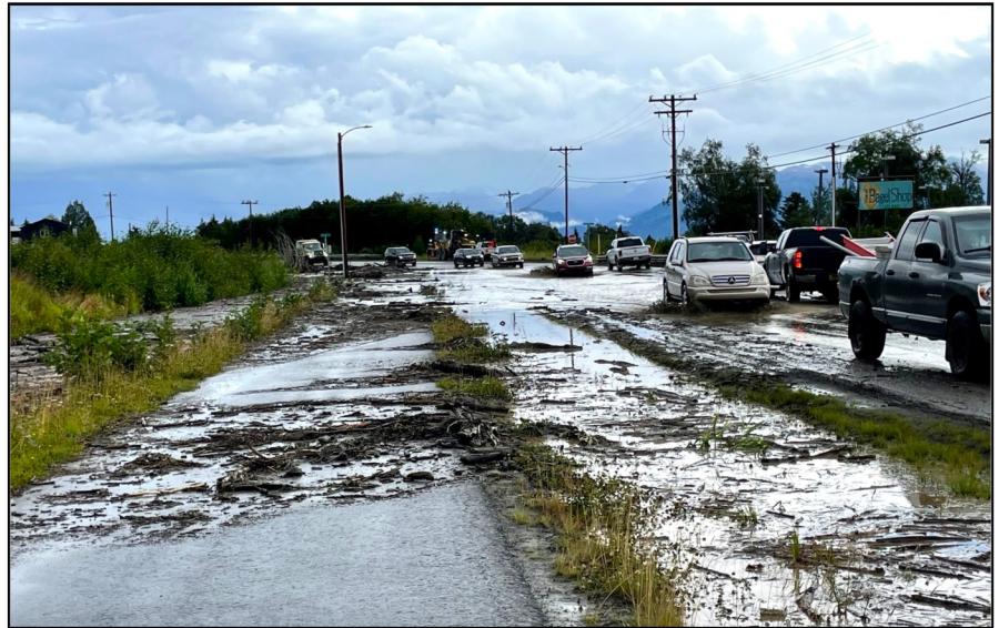
Traffic passing through the flooded section of East End Road at Kachemak Drive.
