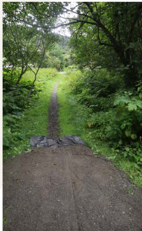
Calhoun resurfacing in progress shows the difference between the old trail and the new one. Photo credit: Matt Steffy
