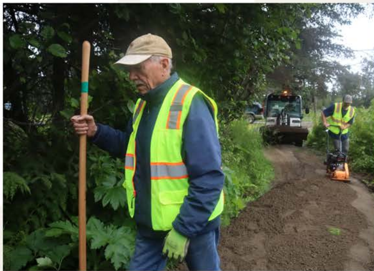
Volunteer Mike Haines smooths out new gravel that City Parks staff Chad Felice delivers with the Toolcat while Matt Hornaday runs the compactor on Calhoun Trail. Photo credit: Matt Steffy
