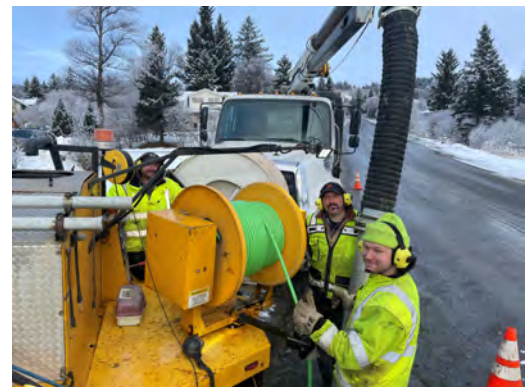
Public Works Utilities crew hard at work! From (R-L) Sean Love, Ralph Skorski and Jason Hanenberger.
