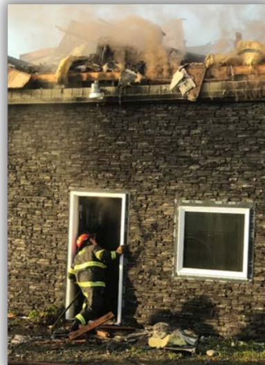
Firefighter checking on smoke location.
