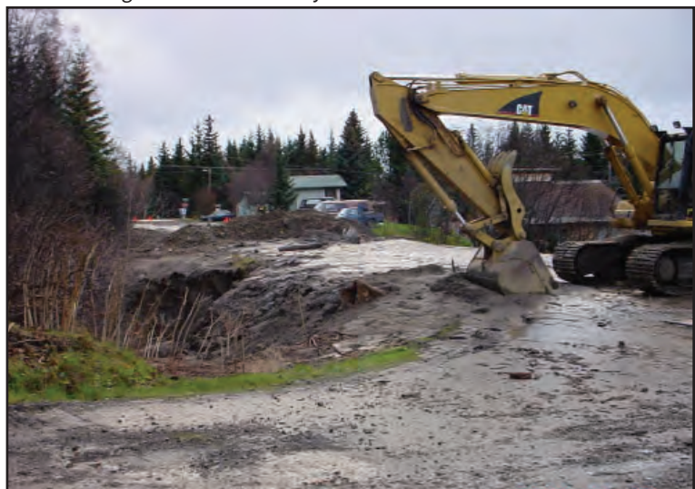
The Slope Stability Program utilizes nature based and low impact development techniques to mitigate erosional damage and protect water quality.
