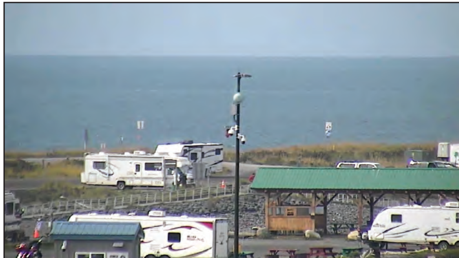
Security cameras, pictured here, center, allow harbor officers to gain situational awareness before responding to an event, to verify details of recorded events and monitor progress of evacuations or check on inundation during tsunami events.
