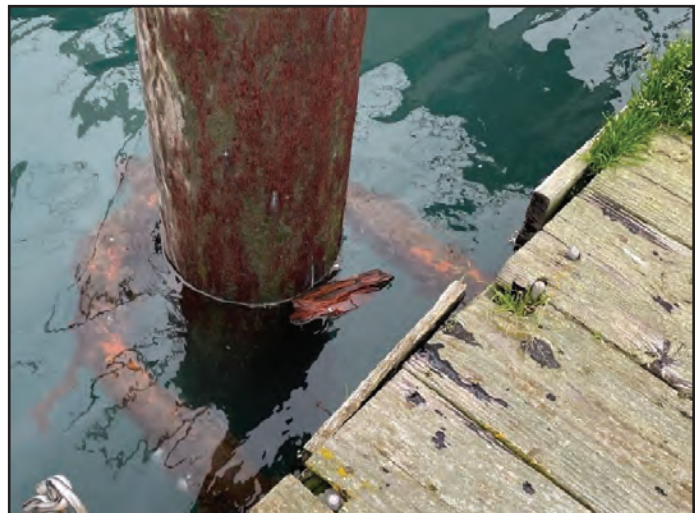
Low freeboard resulting in submerged pile collar. Decking has rot and hardware connections protrude through it.
