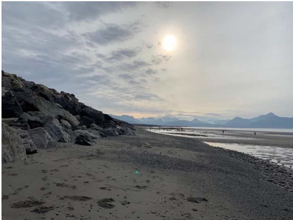
Figure 3. Condition of USACE revetment along the Spit.
