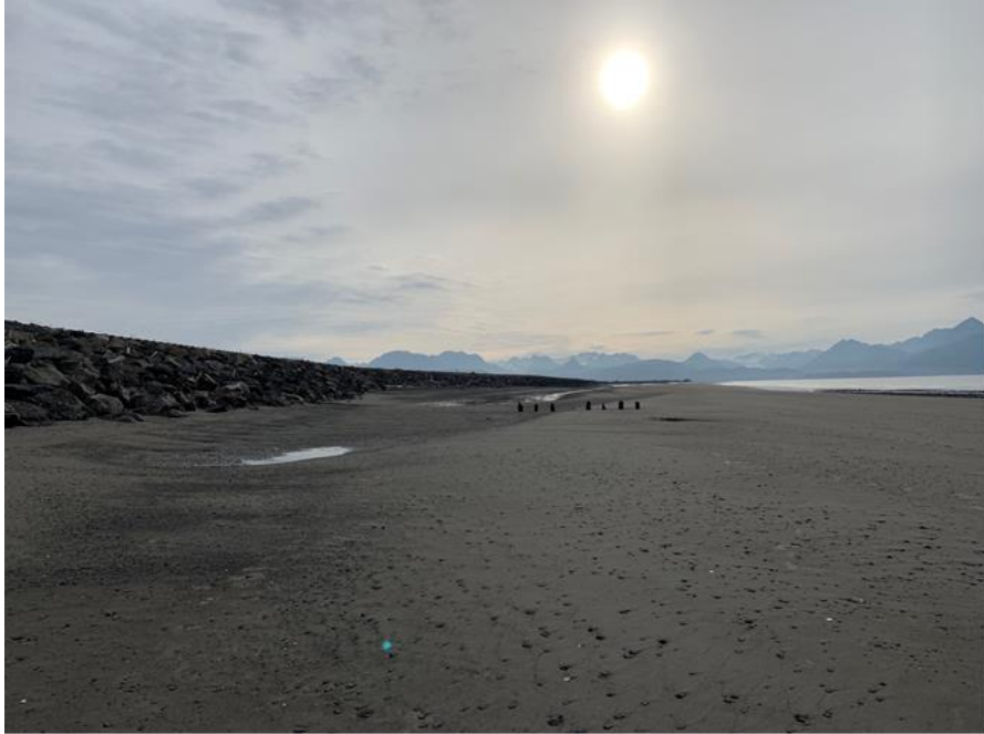
Figure 5. Sand lens observed along DOT&PF revetment.
