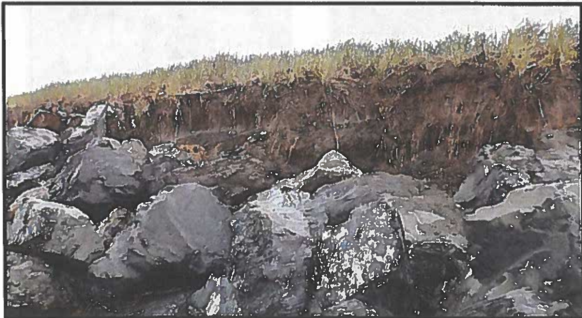
Figure 33. Homer Spit beach nourishment area BN 3, slumping soil at top of the rock transition area and subsequent erosion.
