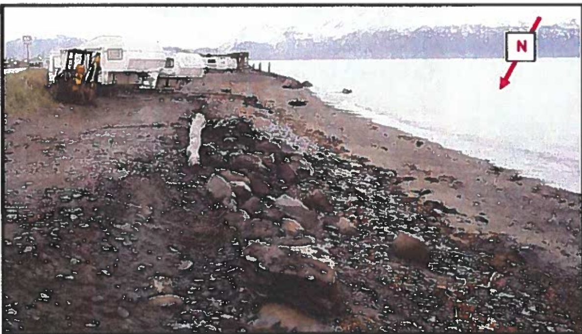
Figure 31. Homer Spit beach nourishment area BN 3, unprotected shoreline extending beyond the rock revetment towards the end of the spit.
