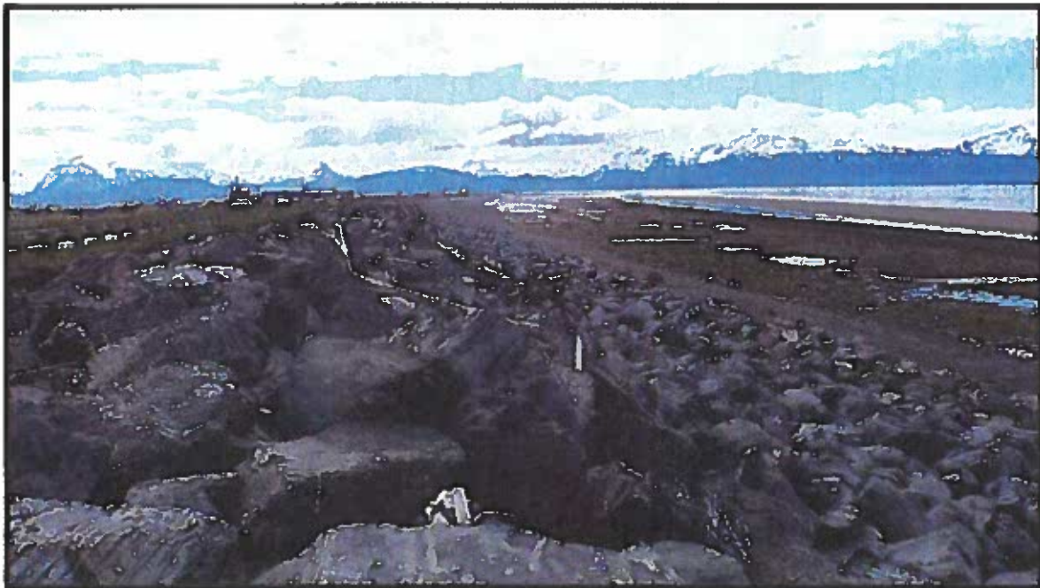
Figure 21. Homer Spit beach nourishment area BN 2, view to southeast, illustrating the rock revetment and offshore topography. Note transition from toe of revetment to gravel beach to band of cobble/tide pools to sand/mud flats.
