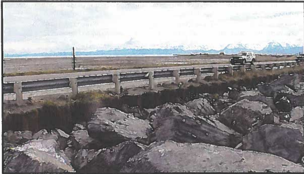
Figure 22. Homer Spit beach nourishment area BN 2, view illustrating rock revetment placement protecting the face of steel sheet pile and Homer Spit Road.
