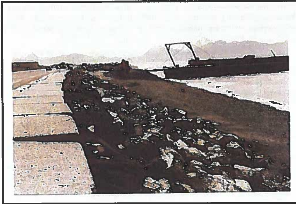
Figure 10. Photograph taken June 18, 1994, when the 1,130 foot long rock revetment was being constructed by the U.S. Army Corps of Engineers. The photograph also shows in the foreground the State of Alaska's 1993 temporary shoreline protection measure which included using pit gravel, concrete blocks, filter fabric, and armor stone to protect the Homer Spit Road.
