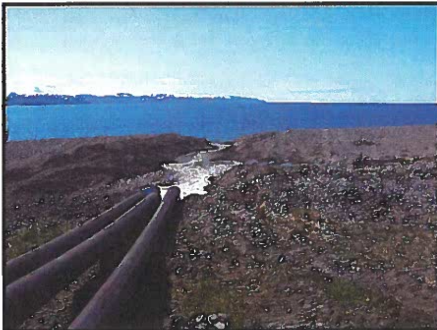
Figure 6. Pipelines from dewatering site leading to beach discharge site, Homer Spit, Alaska
