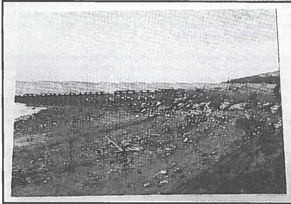
Figure 4. 1963 Photograph of Groyne No. 4 taken in 1963, illustrating the effect of erosion along the down drift and landward end of the groyne, Homer Spit, AK. (Stanley and Grey, 1963).
