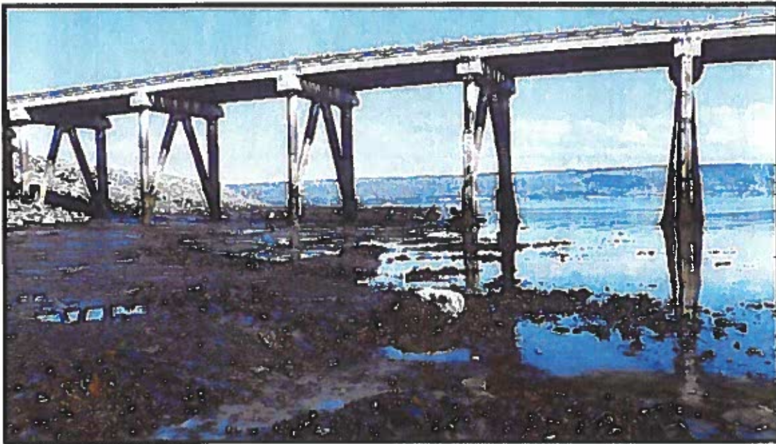
Figure 60. Deep water dock extending through the New Harbor Staging Area disposal site, Homer Spit, AK.
