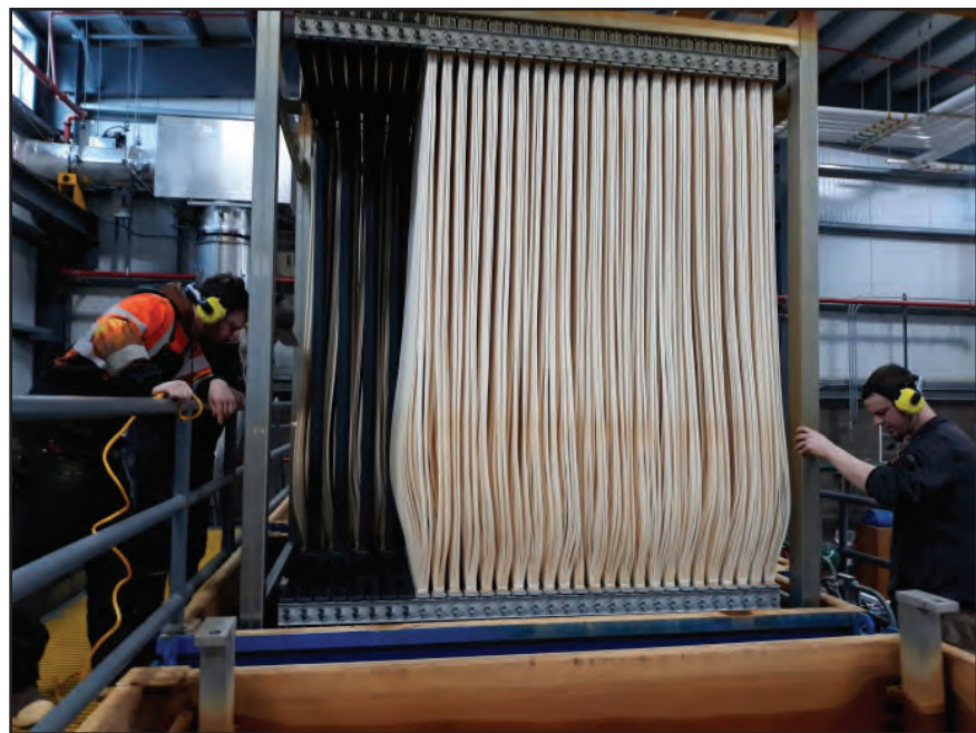
City of Homer Waste Water Treatment Plant staff checking a membrane tray for leaks
