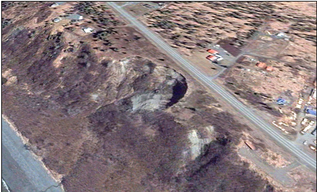
As seen in this aerial image, the eroding edge of the bluff is only 30 feet away from the Sterling Highway at a section just north of Anchor Point.
