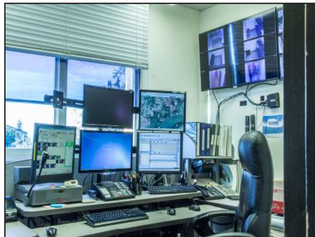
City-wide radio system upgrades are needed to maintain full communication operability.
