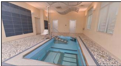
HydroWorx Pool Room .
