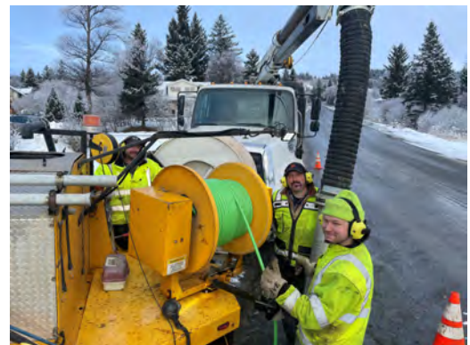
Public Works Utilities crew hard at work! From (R-L) Sean Love, Ralph Skoog, Jason Hanenberger, Page 35 of 44
