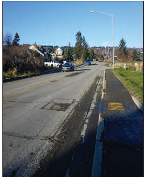
Photo showing the beginning of soft spots mid-way down Heath Street.
