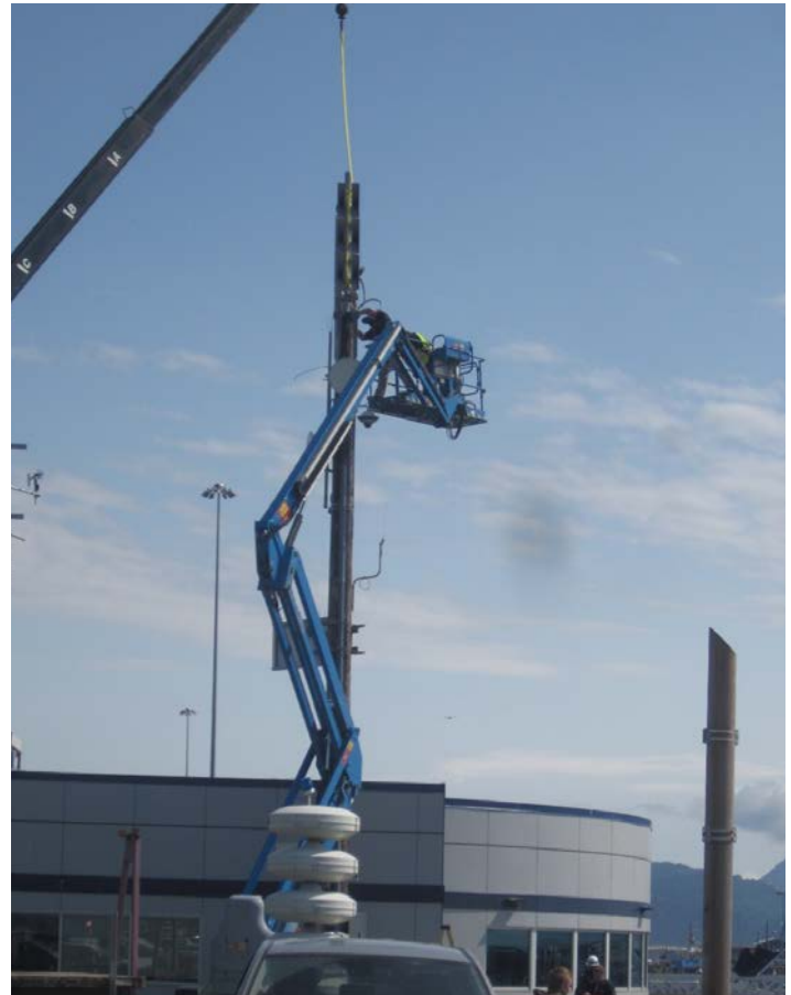
The KPBA's tsunami tower rebuild team installed the new tsunami warning system on the pole next to the Harbormaster's office.
