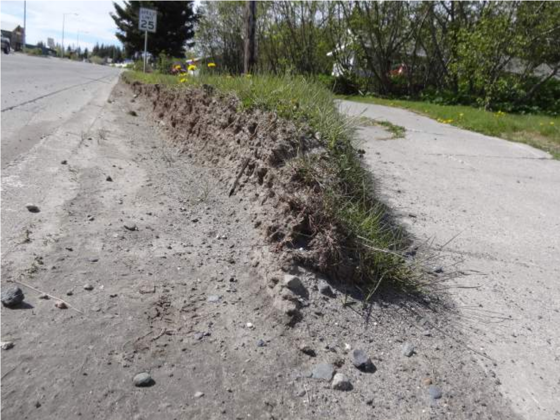
Pics of raised sod between curb and sidewalk on north side of Pioneer in front of Borough office (206 E. Pioneer)
