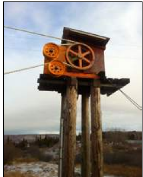
Ohlson Moutain Rope Tow's top station, which supports the engine, bullwheel and weight of the rope in motion, is in need of foundation repair.
