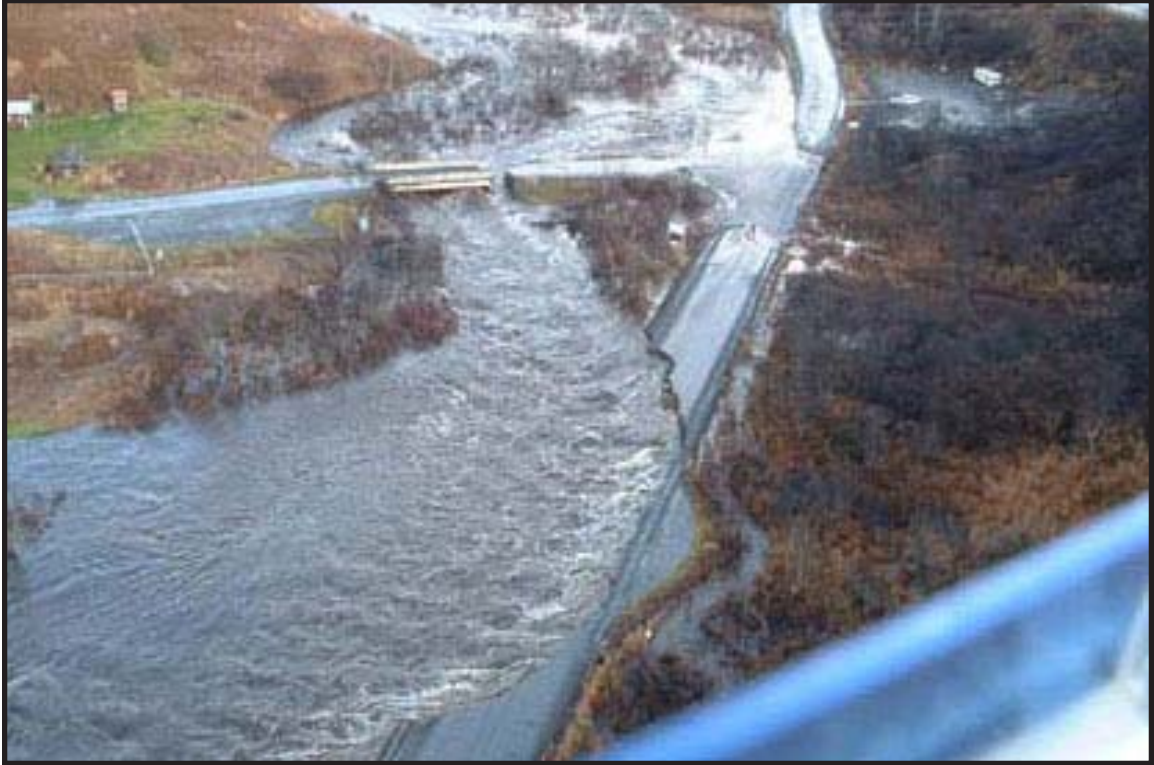
Figure 21. The 2002 flood damaged the bridge over the Ninilchik River and removed much of the road to the spit downstream, delineating the environmental zone in which past land users would likely not have constructed permanent buildings.
