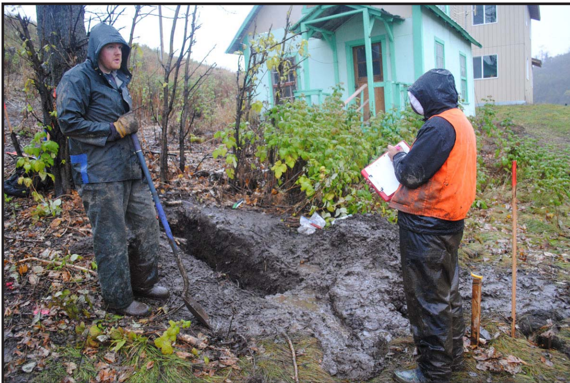
Figure 59. Some mechanically dug as well as hand-dug trenches (such as Trench 45, here looking east) were flooded by groundwater. The soil came out of this trench as a slurry.
