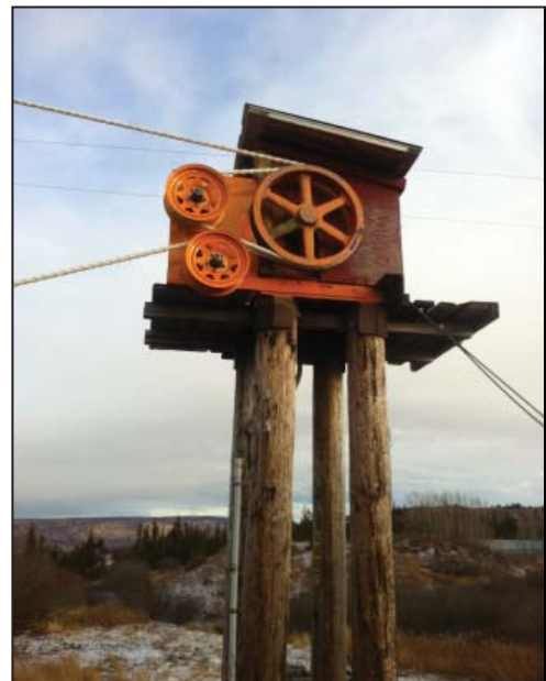
Ohlson Mountain Rope Tow's top station, which supports the engine, bullwheel and weight of the rope in motion, is in need of foundation repair.
